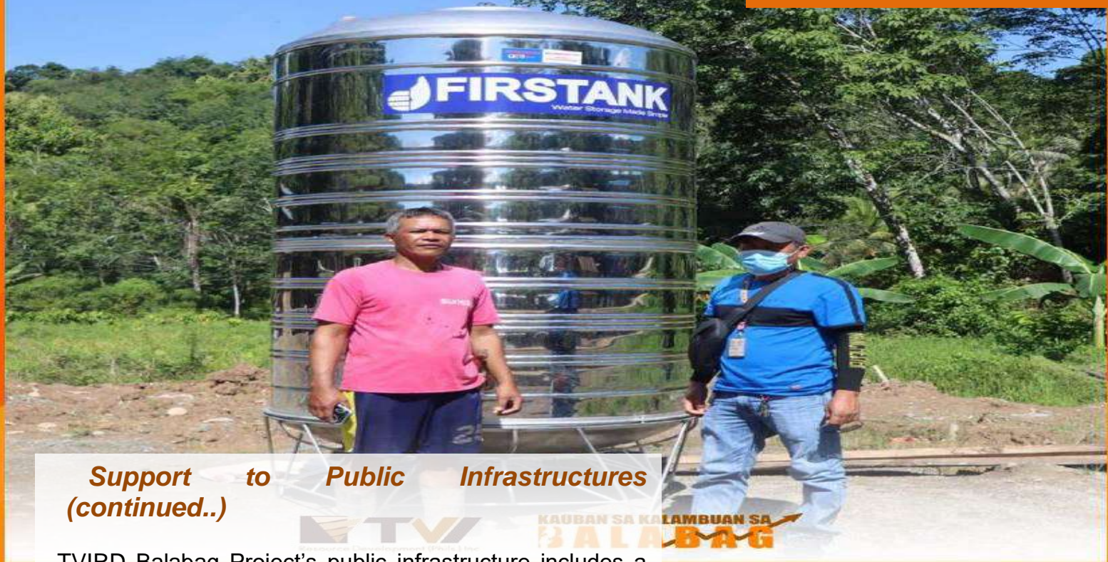
Water Tank turned over to Brgy. Depore
