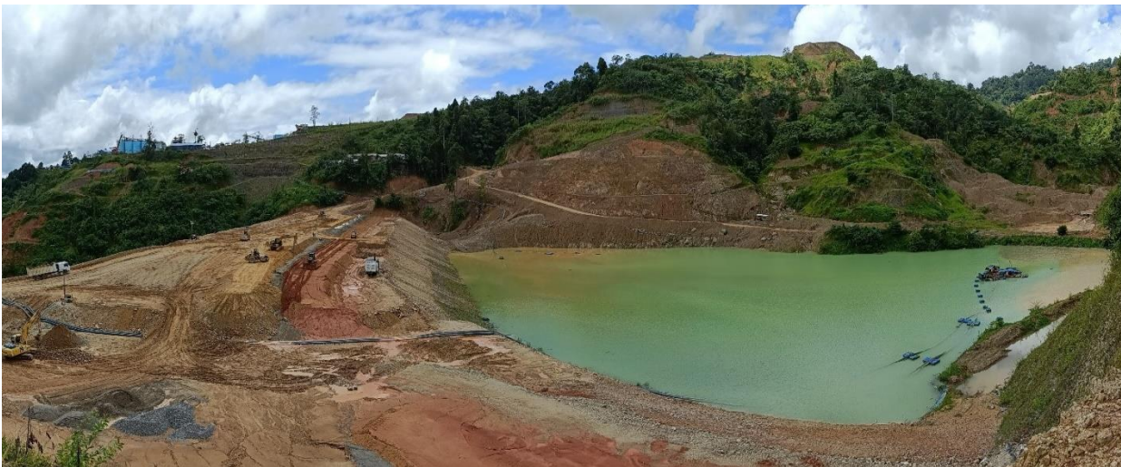
View of TSF on March 27, 2022, looking south from North abutment at RL470m
