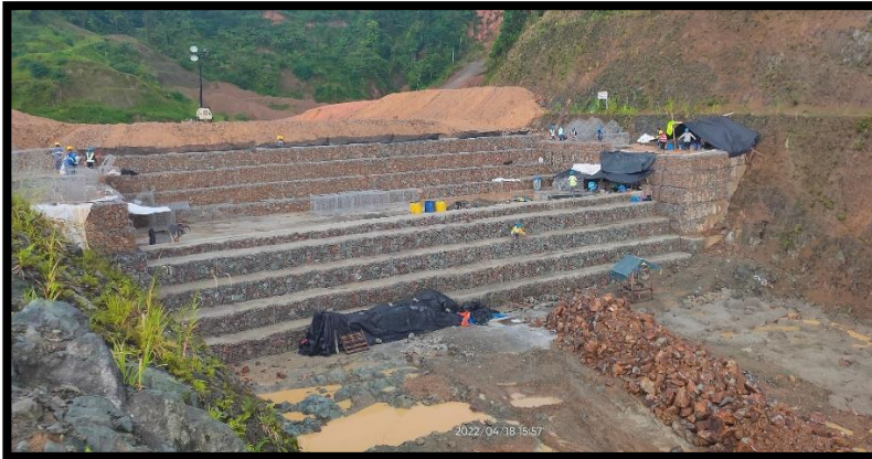
Clearing of diversion channel for concrete backfilling and gabion installation for RL 449 on April 19, 2022.
