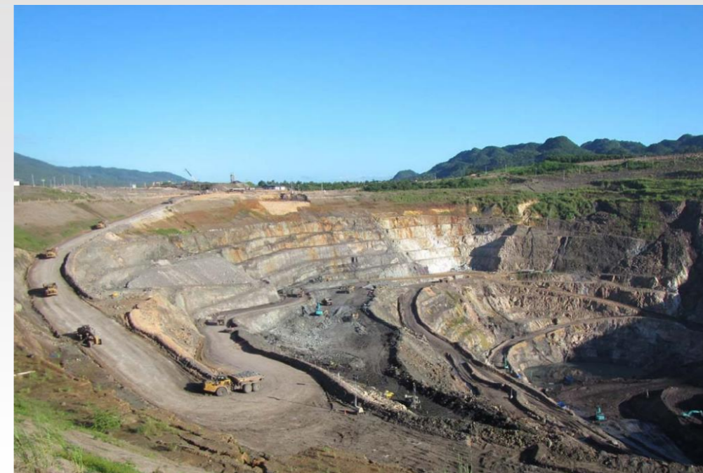
View of the Siana open pit Stage 4 West wall looking north. Source: Red 5 Limited December 2015 Quarterly Activities Report, dated Jan.22.2016.
