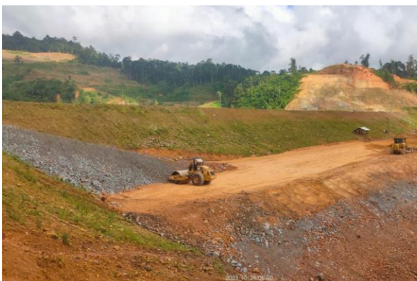
Balabag TSF construction: Stage 3B embankment placement where more than 50% of usable waste has been directed. Photo: October 2023
