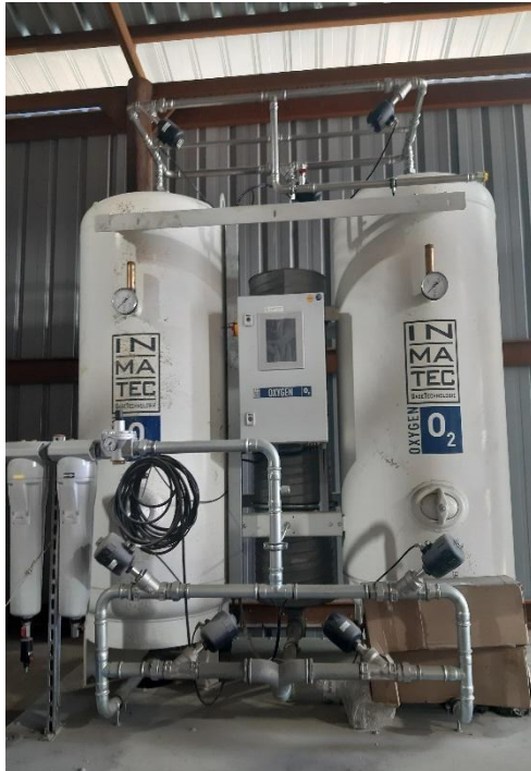
Installation of the oxygen generator in the leaching area of the Balabag Process Plant to further increase the efficiency of the cyanidation process (April 20, 2023).
