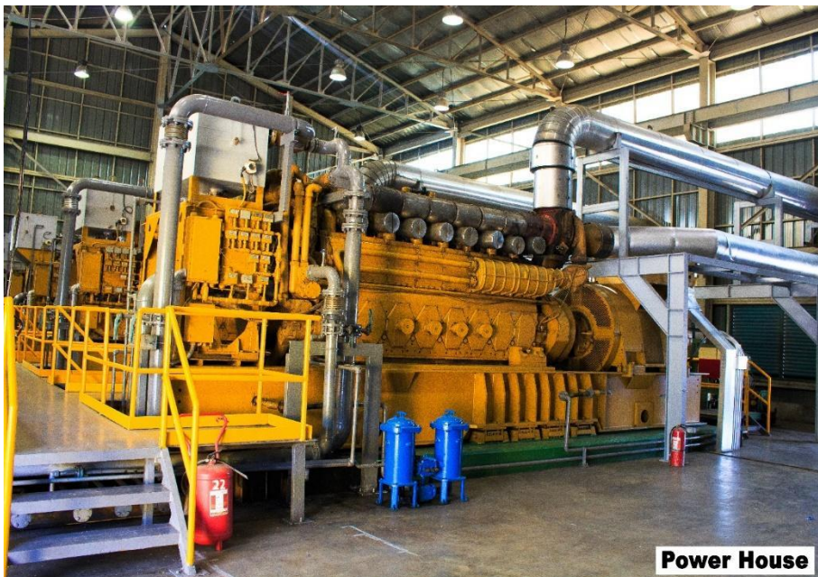
Siana Gold Power House, April 5, 2023
