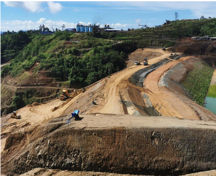
Balabag Tailings Storage Facility Zone 3A placement and embankment works on March 19, 2023.
