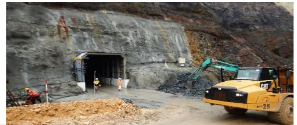
Construction of main access portal at the Siana Underground Mine Source: Red 5 Limited March 2017 Quarterly Activities Report, dated April 28, 2017.
