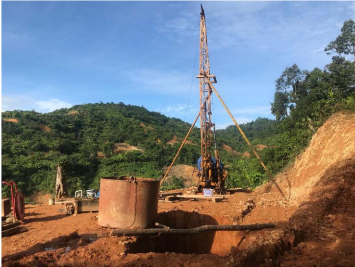
Location of drill area for Borehole no.1. EDCO started with the SPT in preparation for packer test
