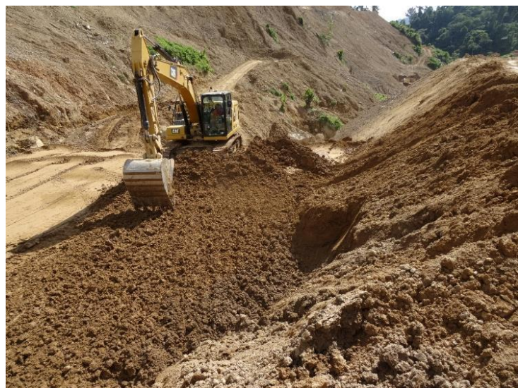
Excavator scarifying the Cofferdam surface prior to compaction. The surface was sealed with a smooth drum compactor due to impending rainfall.
