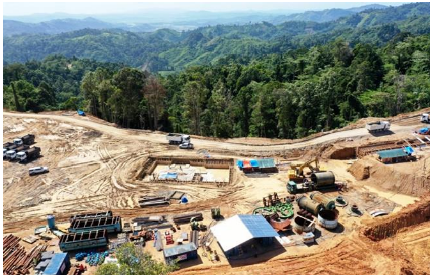
Aerial view of proposed Mill Plant Site of the Balabag Gold Project, showing two ball mills, the SAG Mill, flotation cells, and two tanks, following their arrival from Canatuan
