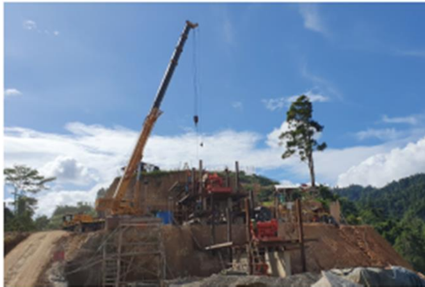
Crushing Circuit: Primary Jaw Crusher Base
