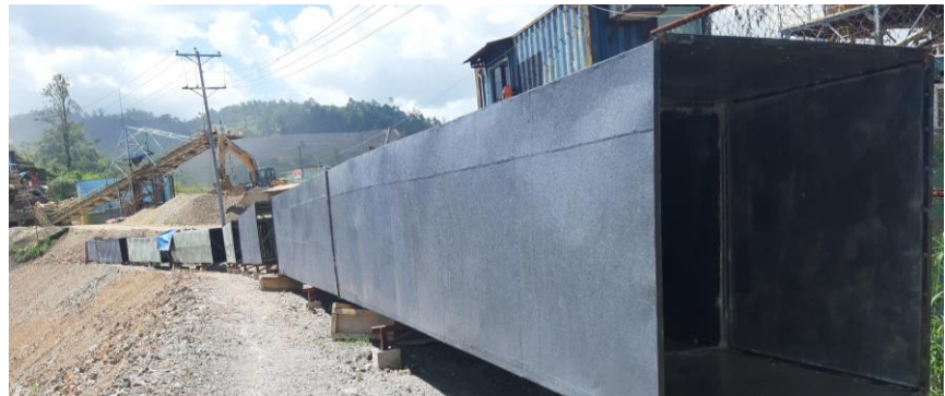
Construction of ductwork system for all fume stack to reduce exposure of genset to fumes and improve equipment reliability.
