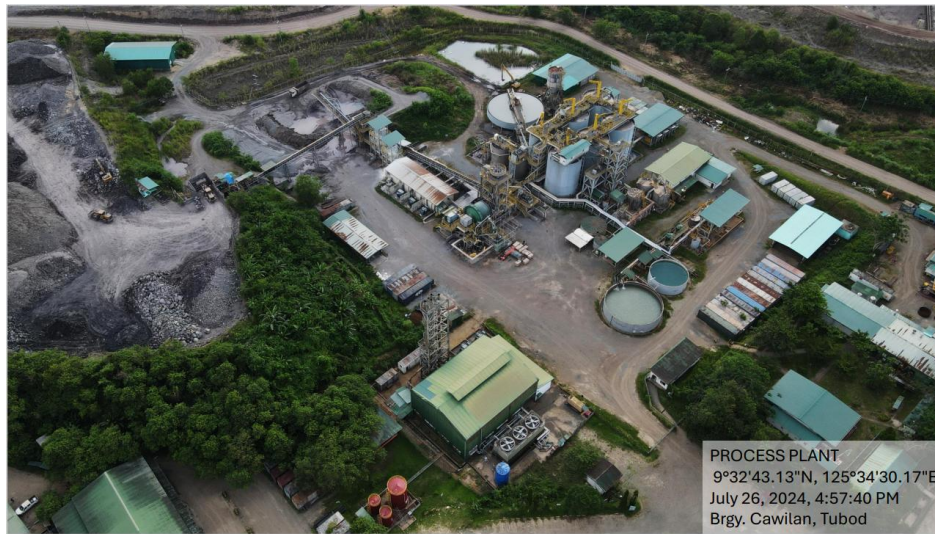
Photo of the Siana Process Plant Facilities (July 26, 2024)
